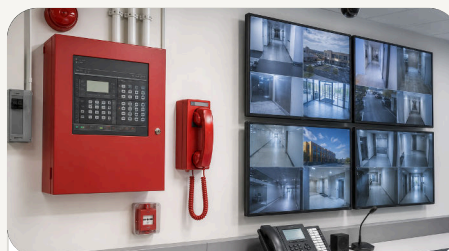
CCTV Systems & Fireman Telephone Systems
